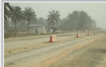
Reconstruction of Odukpani -Itu-Ikot Ekpene Road, Cross River state (Section 1 - Odukpani-Itu Bridge)
